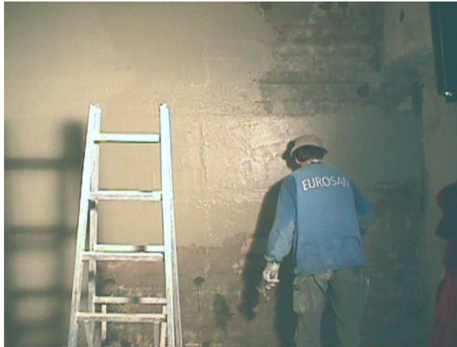
Restoration and waterproofing work on extensive wet, salt-loaded concrete walls of an underground car park with Cembond®M-945.
