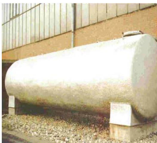
Storage tank insulated with PUR foam and coated with protective coating.
